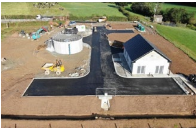
Ardfinnan Regional Water Supply Scheme - Ballylooby Springs
