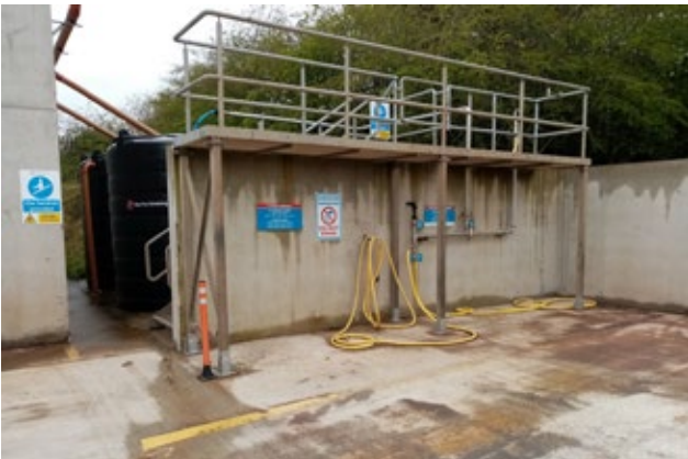
Rainwater Harvesting Unit for Washing Salting Trucks
