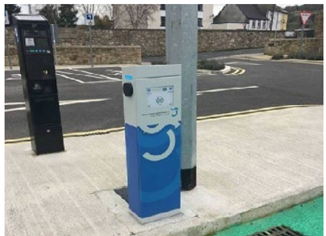
EV Car Charging in Clonmel
