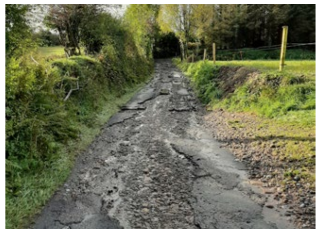
Road Damage Caused by Flooding Event October 2019
