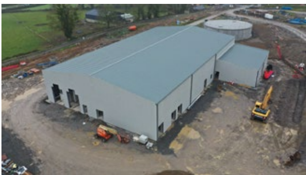
Thurles Water Treatment Plant
