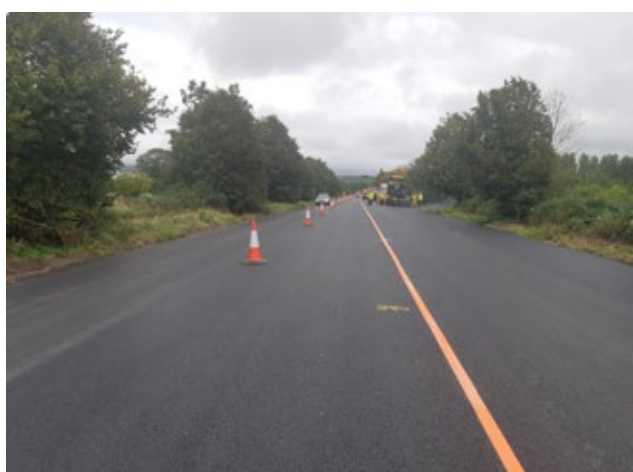
Works in progress on the R445 - Nenagh to Toomevara (former national road)
