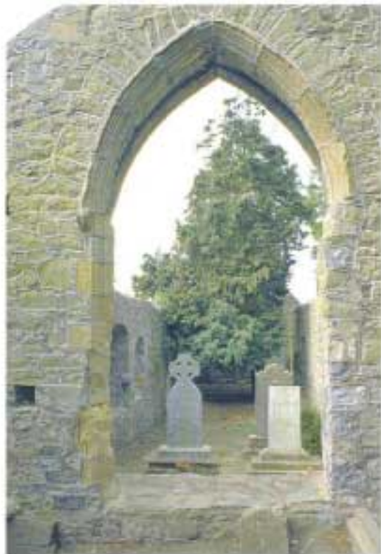
Above: The use of cement mortar and ribbon pointing, as shown here, is inappropriate in the conservation of medieval buildings.
