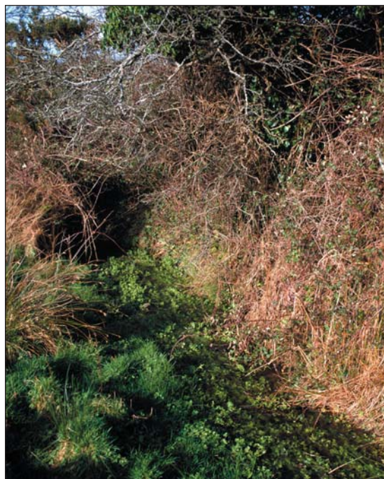
Stream overgrown with vegetation which requires dredging to reduce risk of flooding
