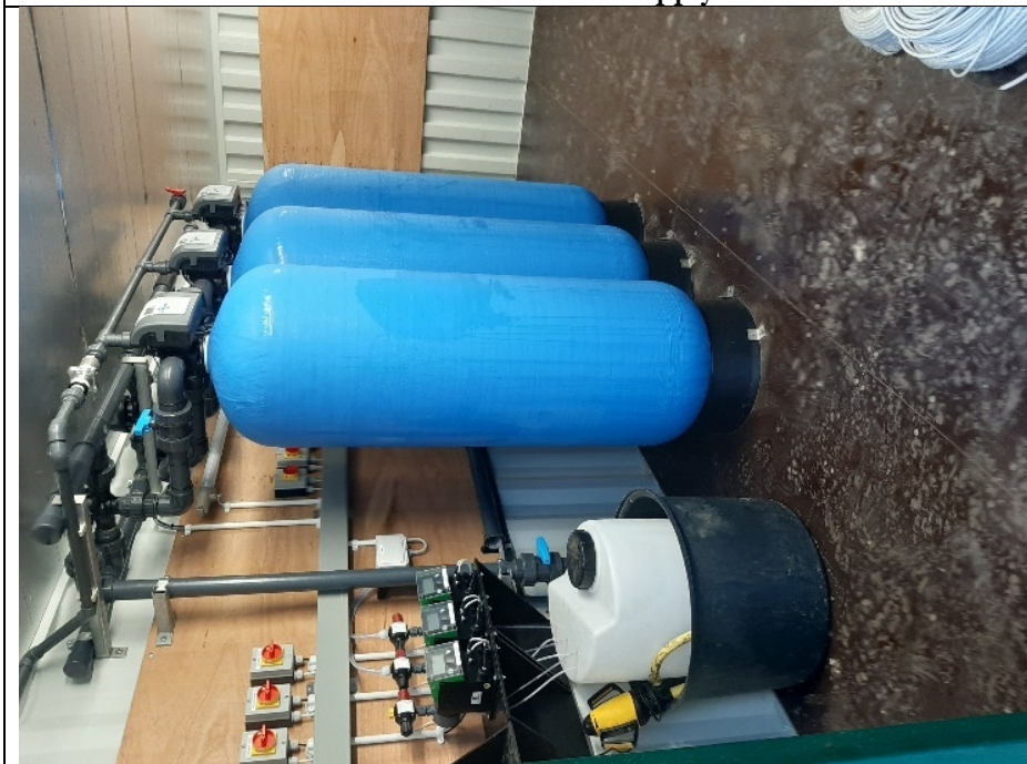
Dualla Public Water Supply
