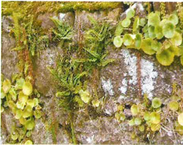
Stone walls with small crevices or lime mortar can support wall plants including certain ferns that only grow on exposed rock
