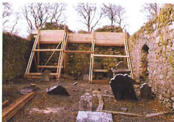
Ongoing conservation works with timber bracing used to support a masonry wall temporarily at Stradbally, Co. Waterford
