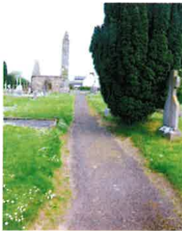
Tarmac pathways can become dangerous as they deteriorate over time
