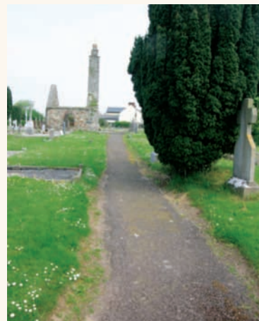
Tarmac pathways can become dangerous as they deteriorate over time
