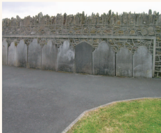
At this graveyard, memorials have been removed from their original location and placed against a graveyard wall. The heavy ribbon pointing of the graveyard wall should also be avoided
