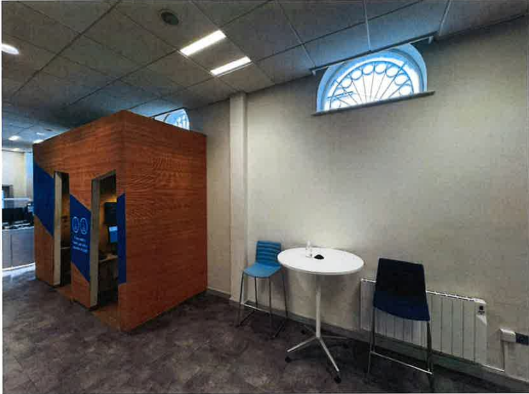
Plate 8: View of the internal face of wall onto which the defibrillator unit will be affixed.
