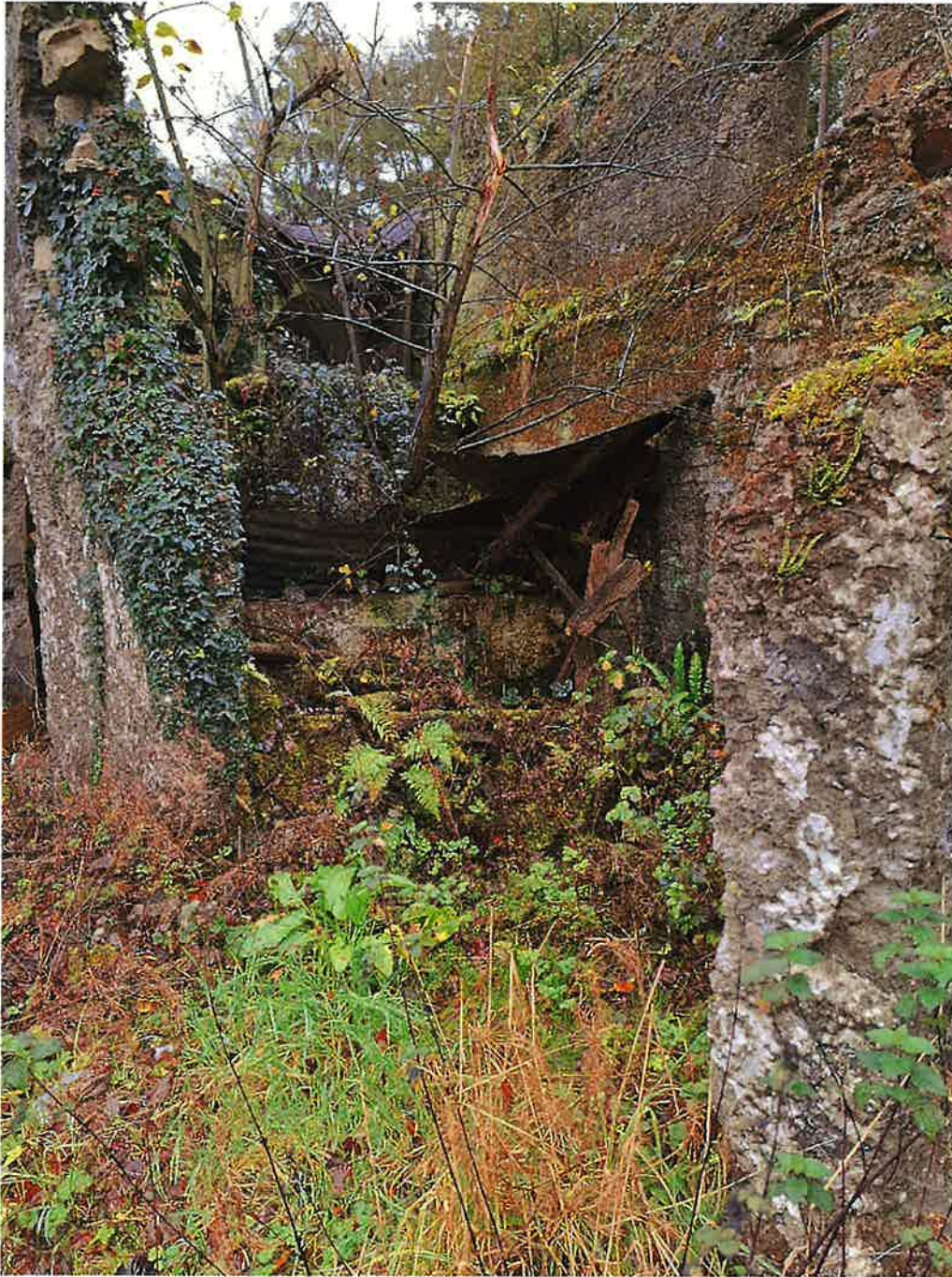
View Into derelict section- Marked P01 on drawing P04
