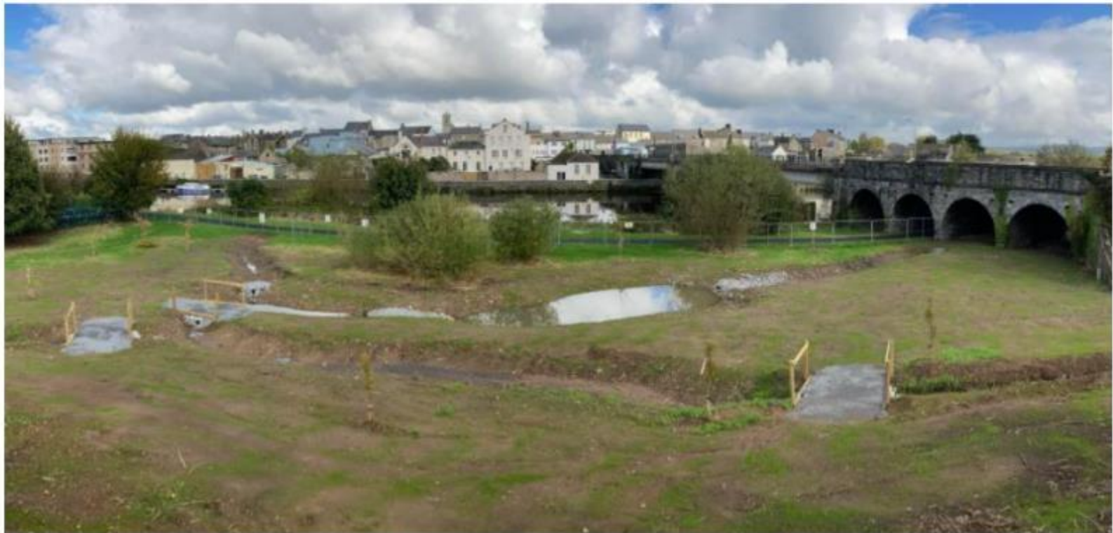
The water treatment pods and vegetated swales created at the Bog Field at Carrickbeg,
