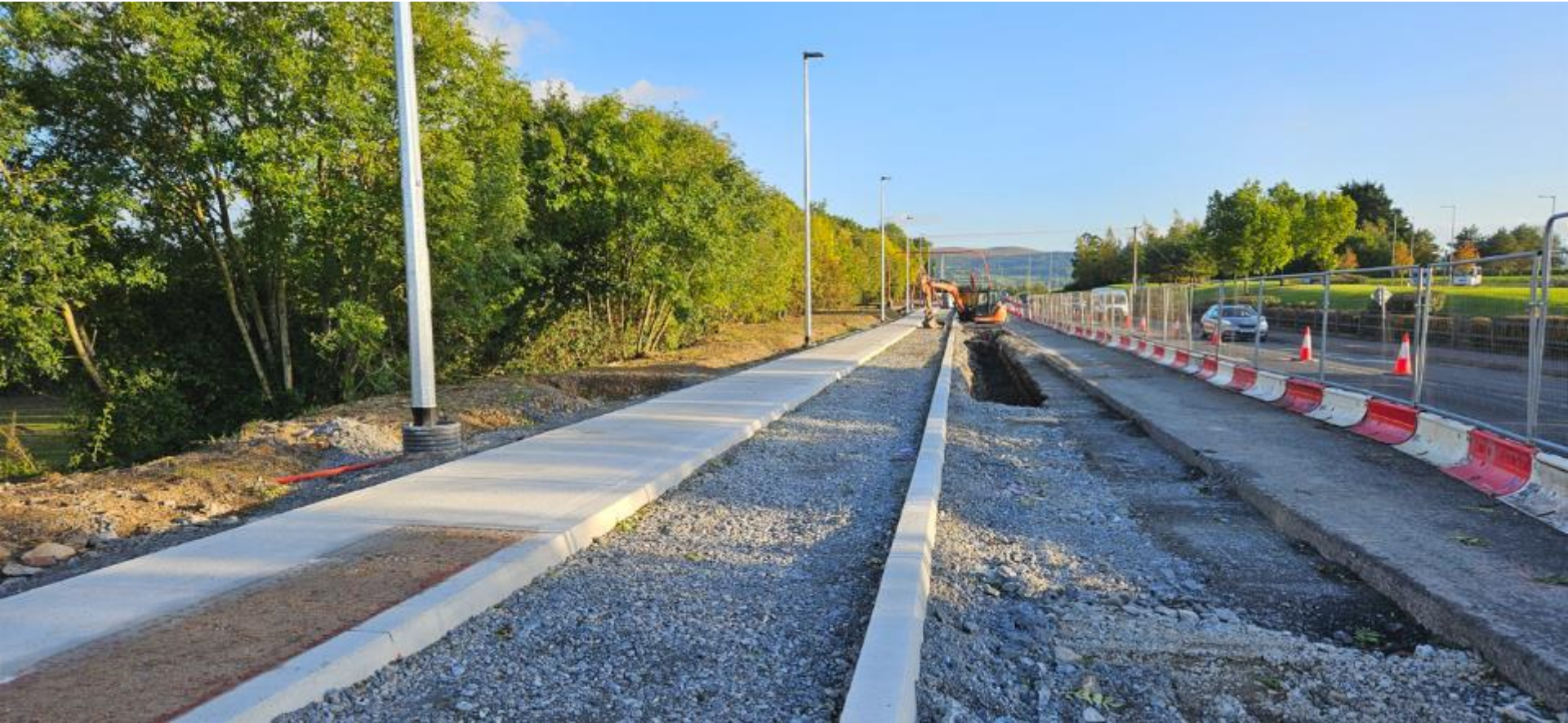
Bioretention Areas (Rain Gardens) – Clonmel
