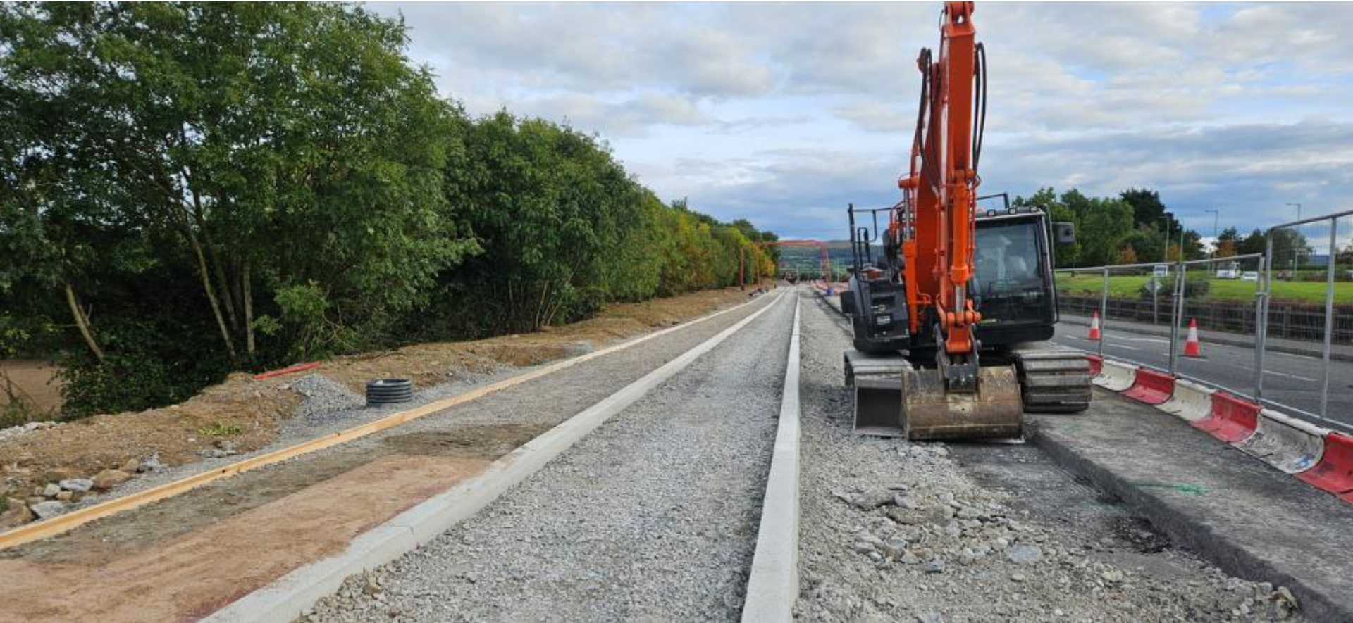
Bioretention Areas (Rain Gardens) – Clonmel
