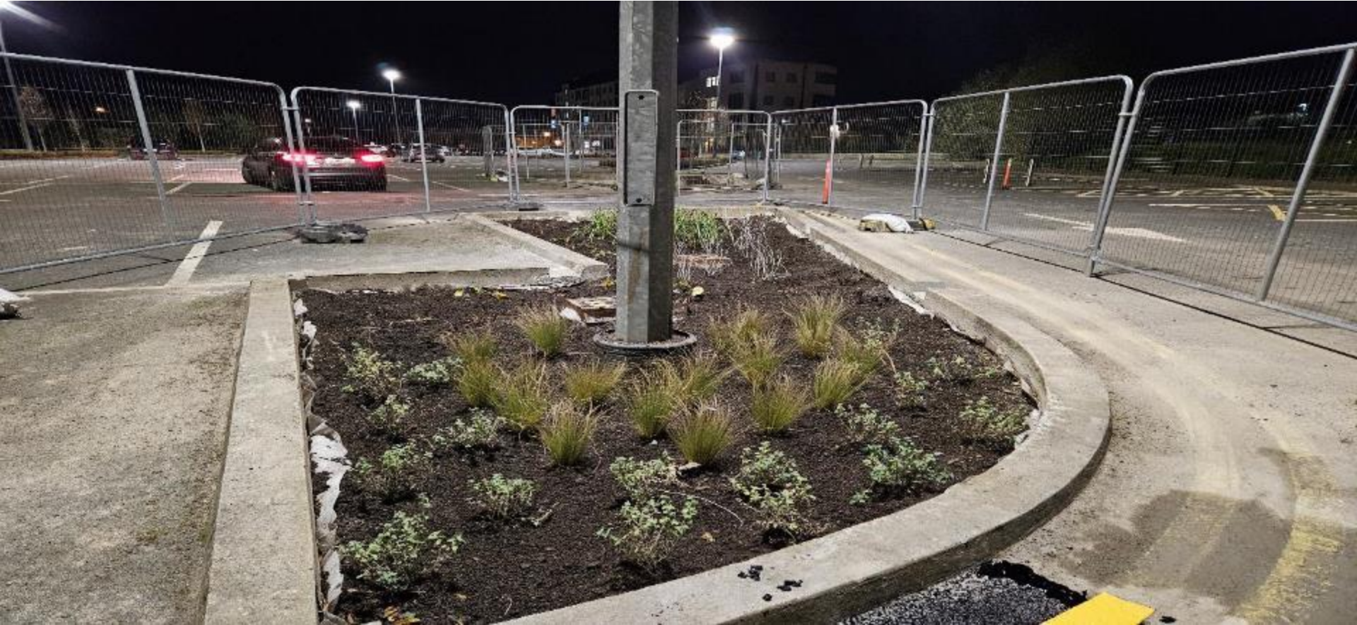
Bioretention Areas (Rain Gardens) – Clonmel
