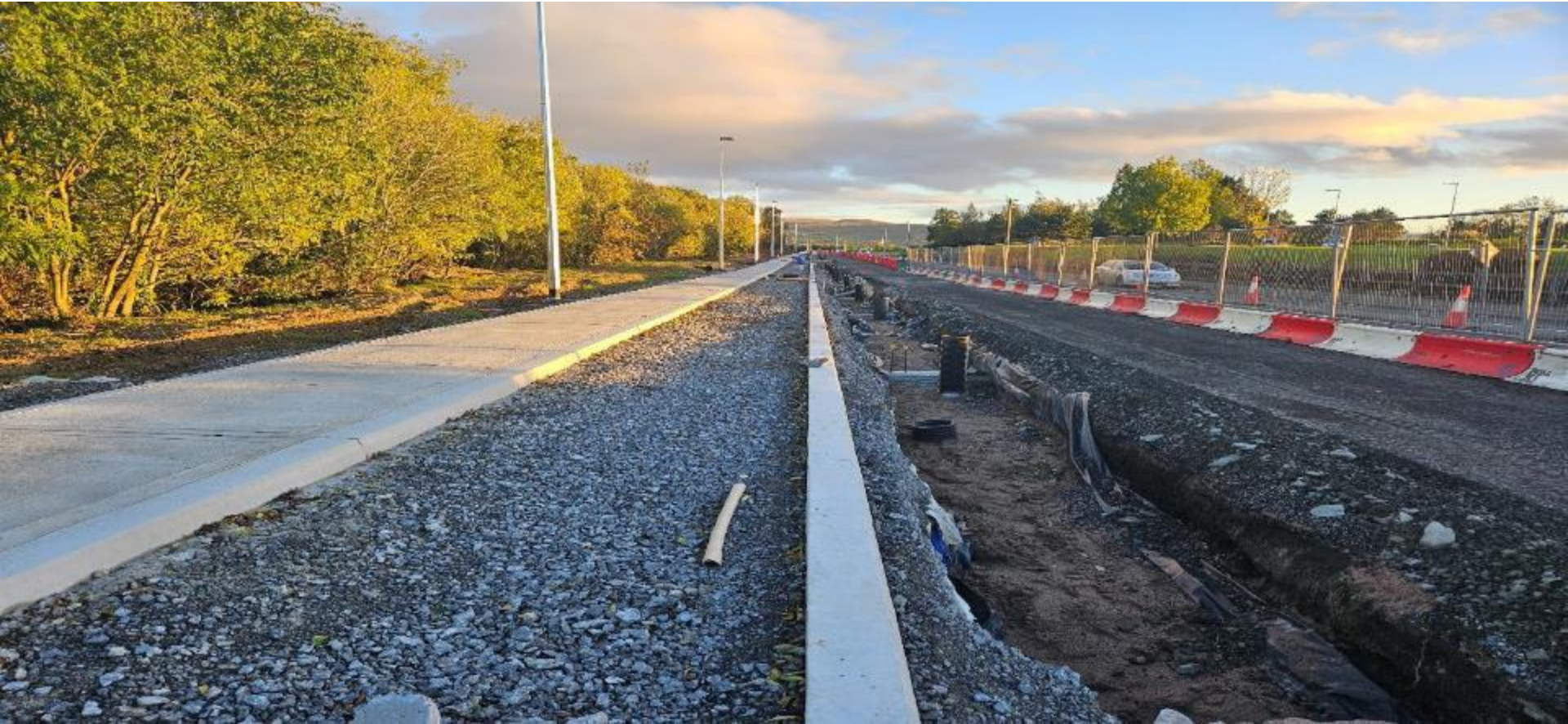
Bioretention Areas (Rain Gardens) – Clonmel
