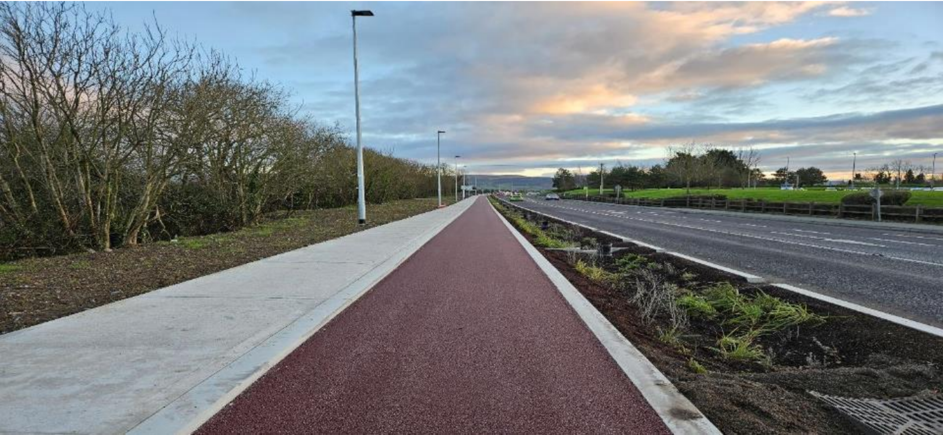
Bioretention Areas (Rain Gardens) – Clonmel
