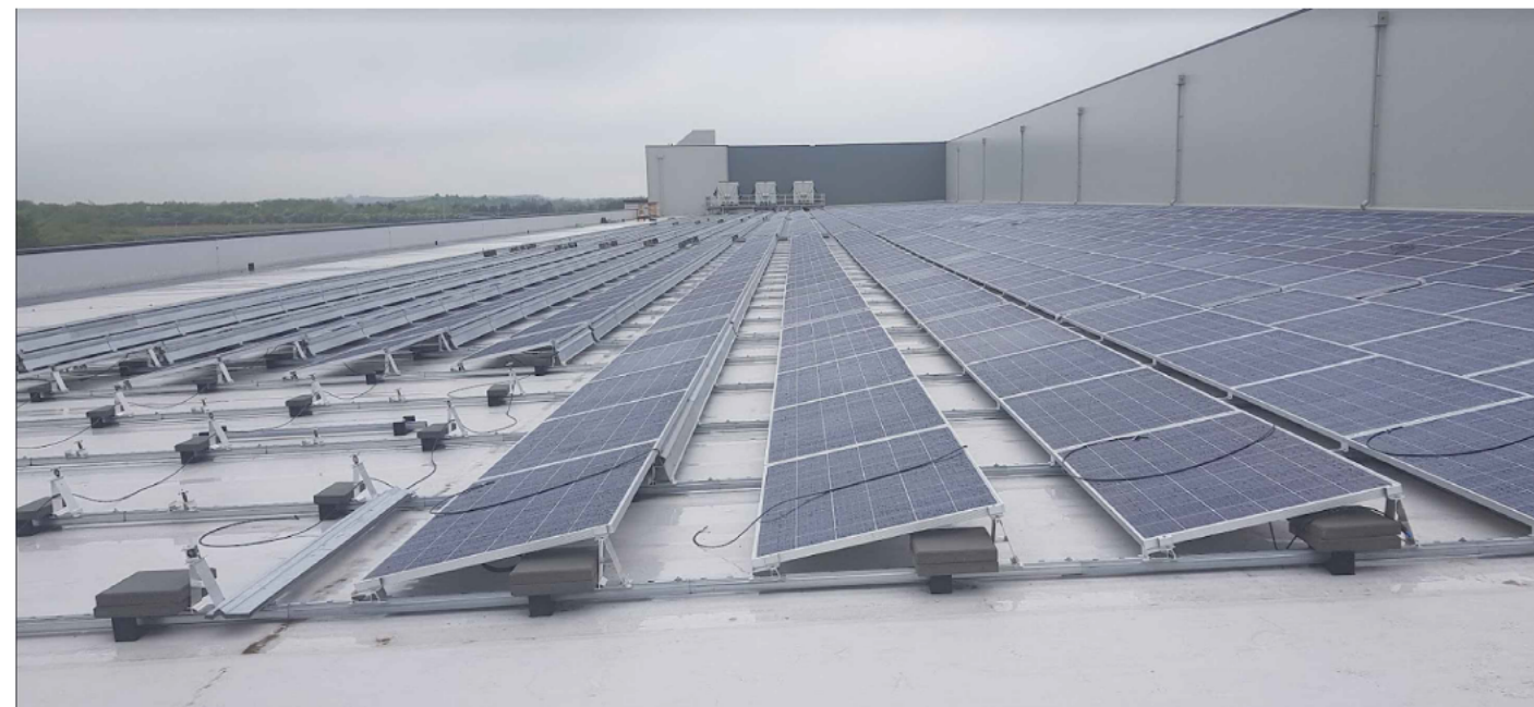
Image of typical PV array (south facing)
