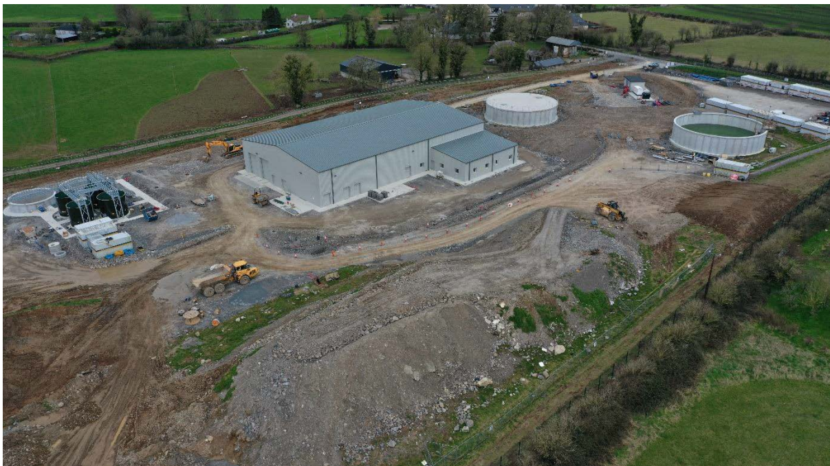
Thurles Regional Water Supply Scheme - Water Treatment Plant
