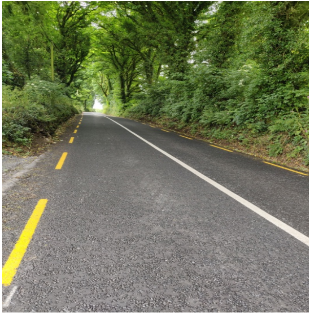
R503 Shevry, recent overlay using HRA (Hot Rolled Asphalt)
