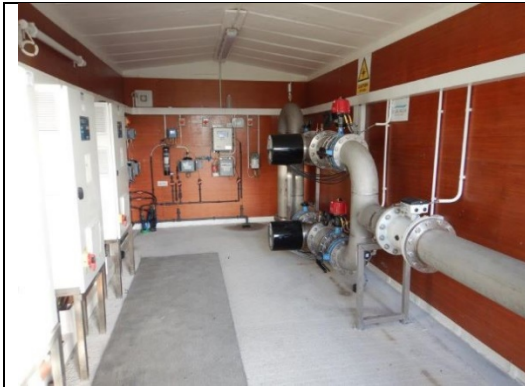
Disinfection Upgrade at Monroe Water Treatment Plant, Clonmel
