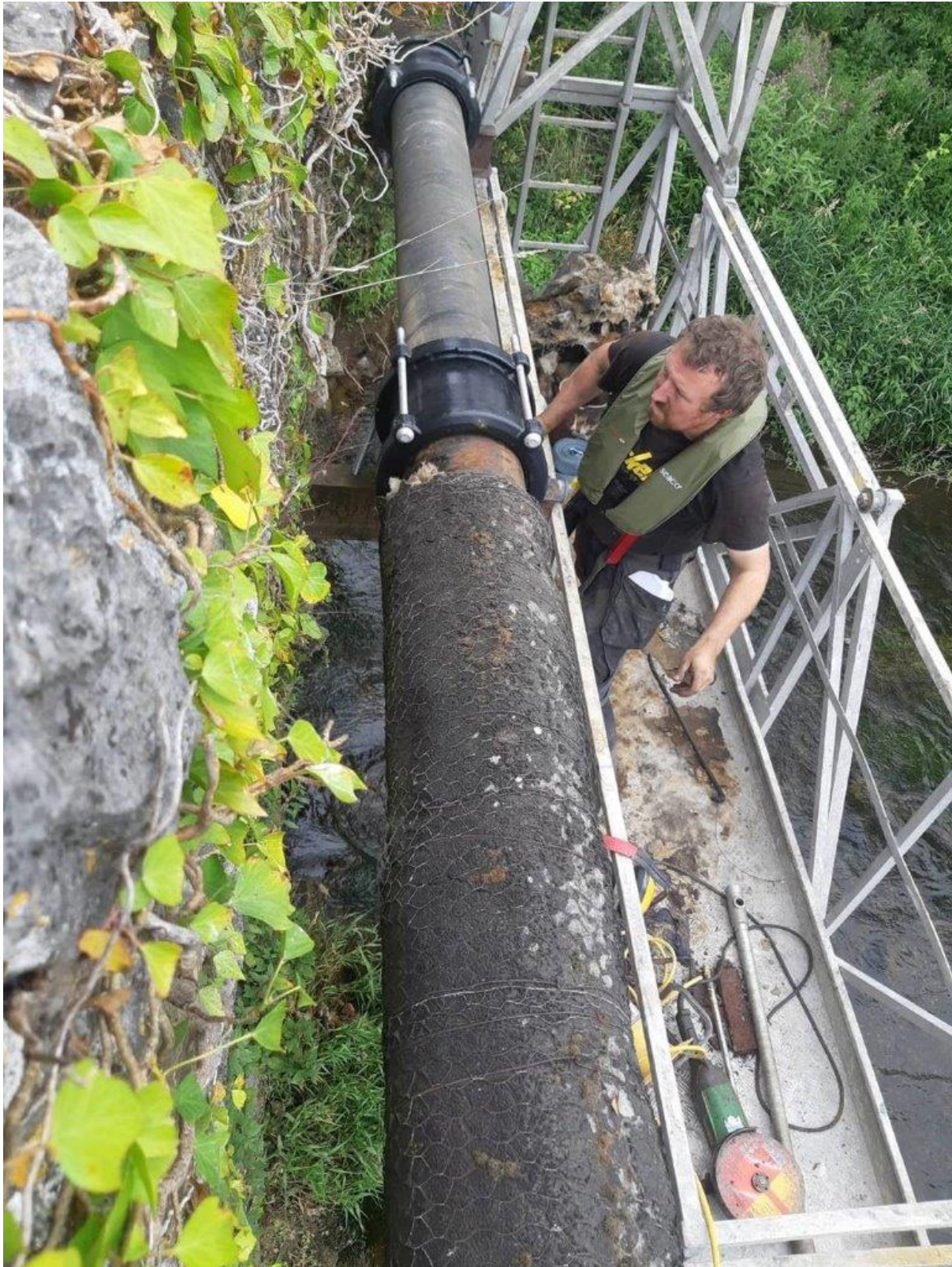
Watermain repairs at New Bridge (also known as Suirville Bridge), Ballycarron, Golden
