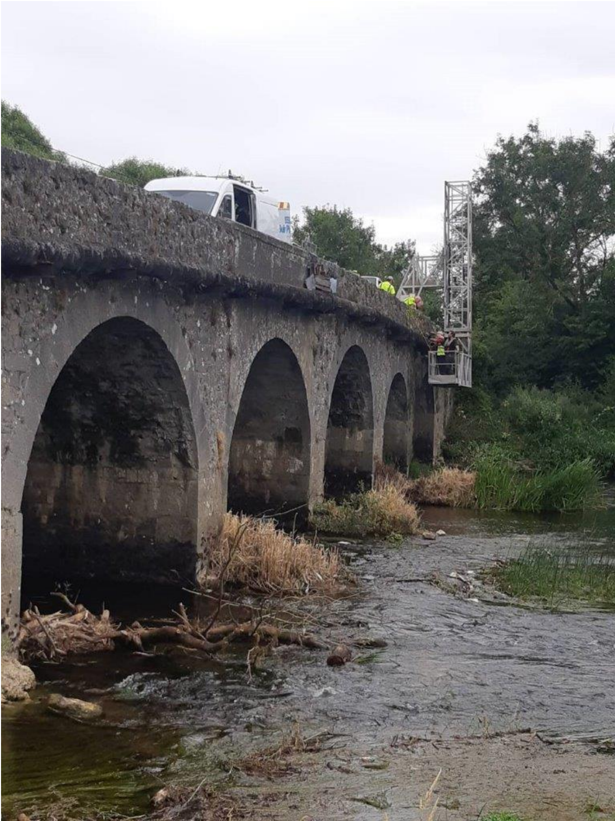
Watermain repairs at New Bridge (also known as Suirville Bridge), Ballycarron, Golden
