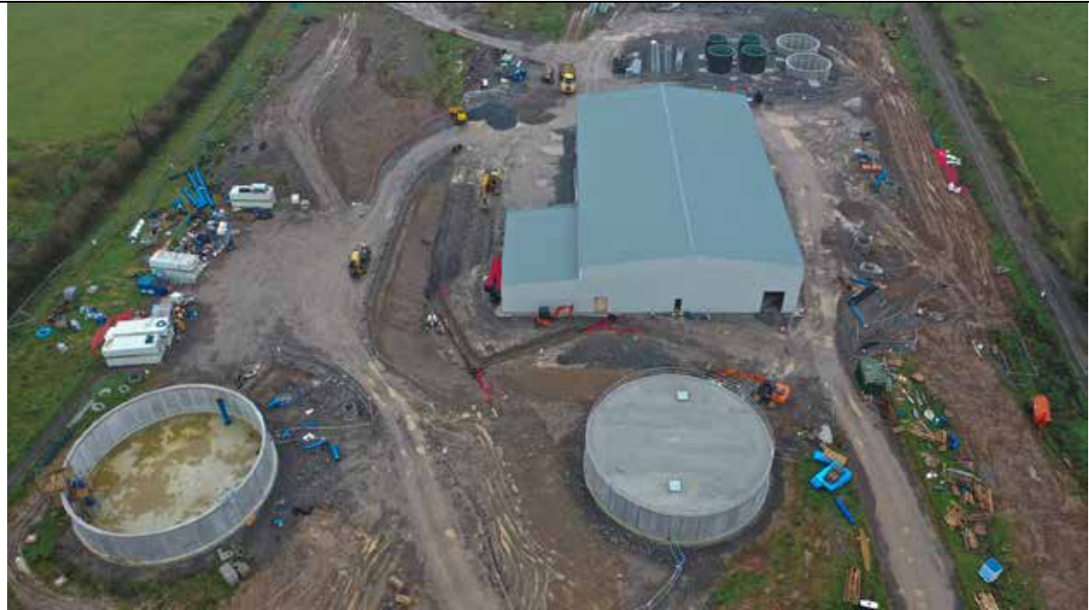
Photograph No. 4: Thurles Regional Water Supply Scheme water treatment plant at Bohernacrusha, Holycross, Thurles.
