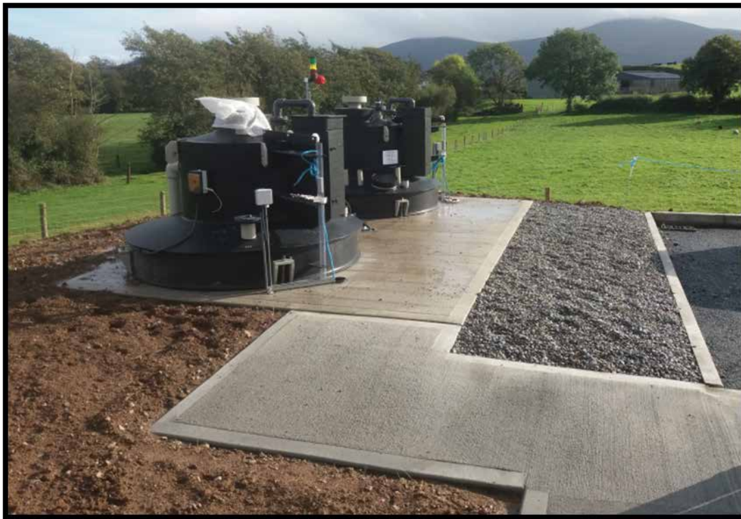
Photograph No. 2: Ardfinnan Regional Water Supply Scheme water treatment plant at Scart East, Ballylooby, Cahir.
