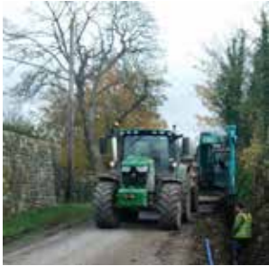
Figure 1: Interconnection Watermain at Plunket Street - Gurteenakilla Group Water Scheme: the civil works providing this interconnection watermain have been completed.
