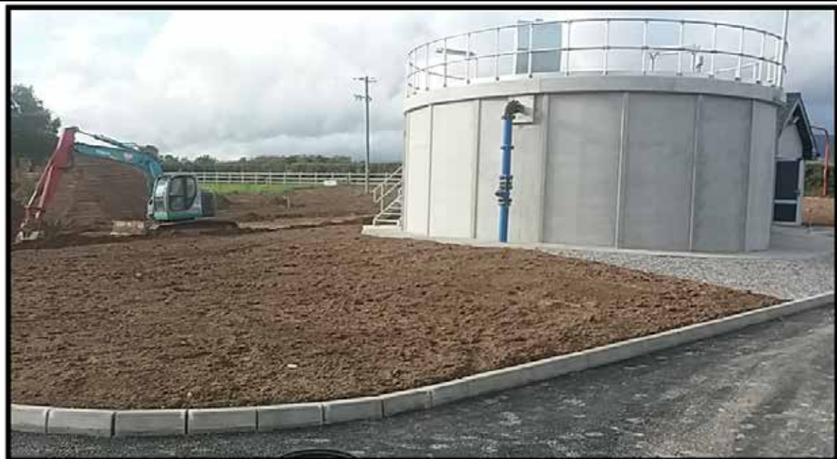
Photograph No. 3: Ardfinnan Regional Water Supply Scheme water treatment plant at Scart East, Ballylooby, Cahir.
