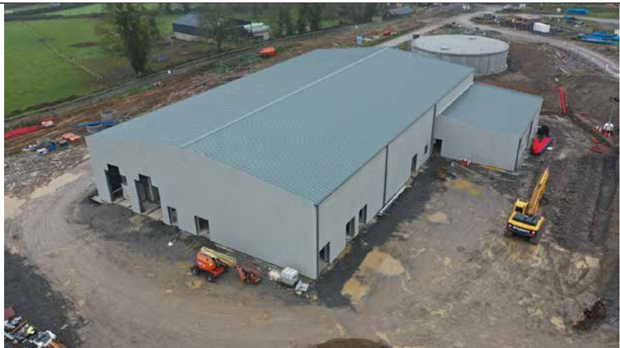
Photograph No. 5: Thurles Regional Water Supply Scheme water treatment plant at Bohernacrusha, Holycross, Thurles.
