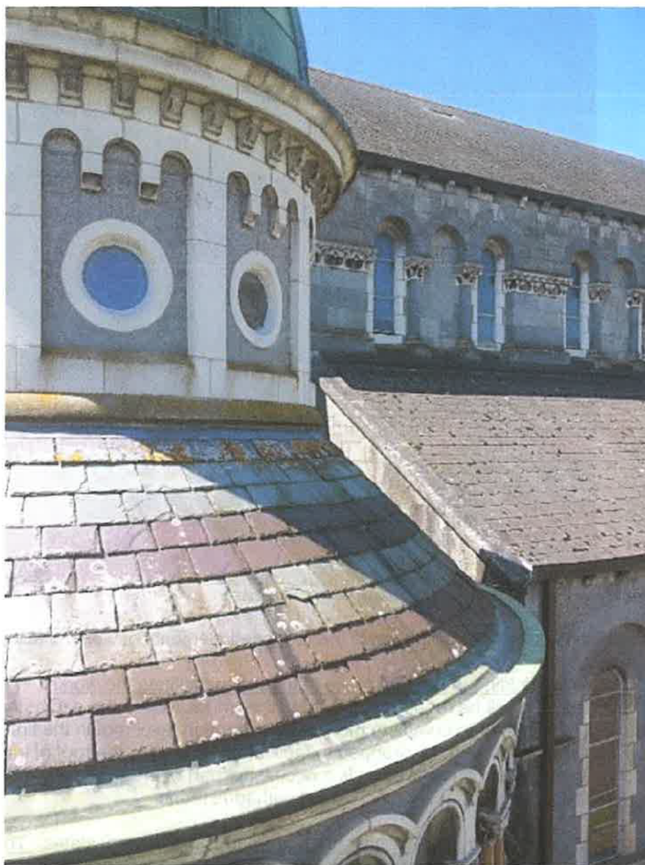
Fig. 6 Detail of roof of baptistry with surviving bands of nineteenth century Bangor blue and Killaloe grey natural slate. The fibre cement slates of the east side aisle are visible in the background.
