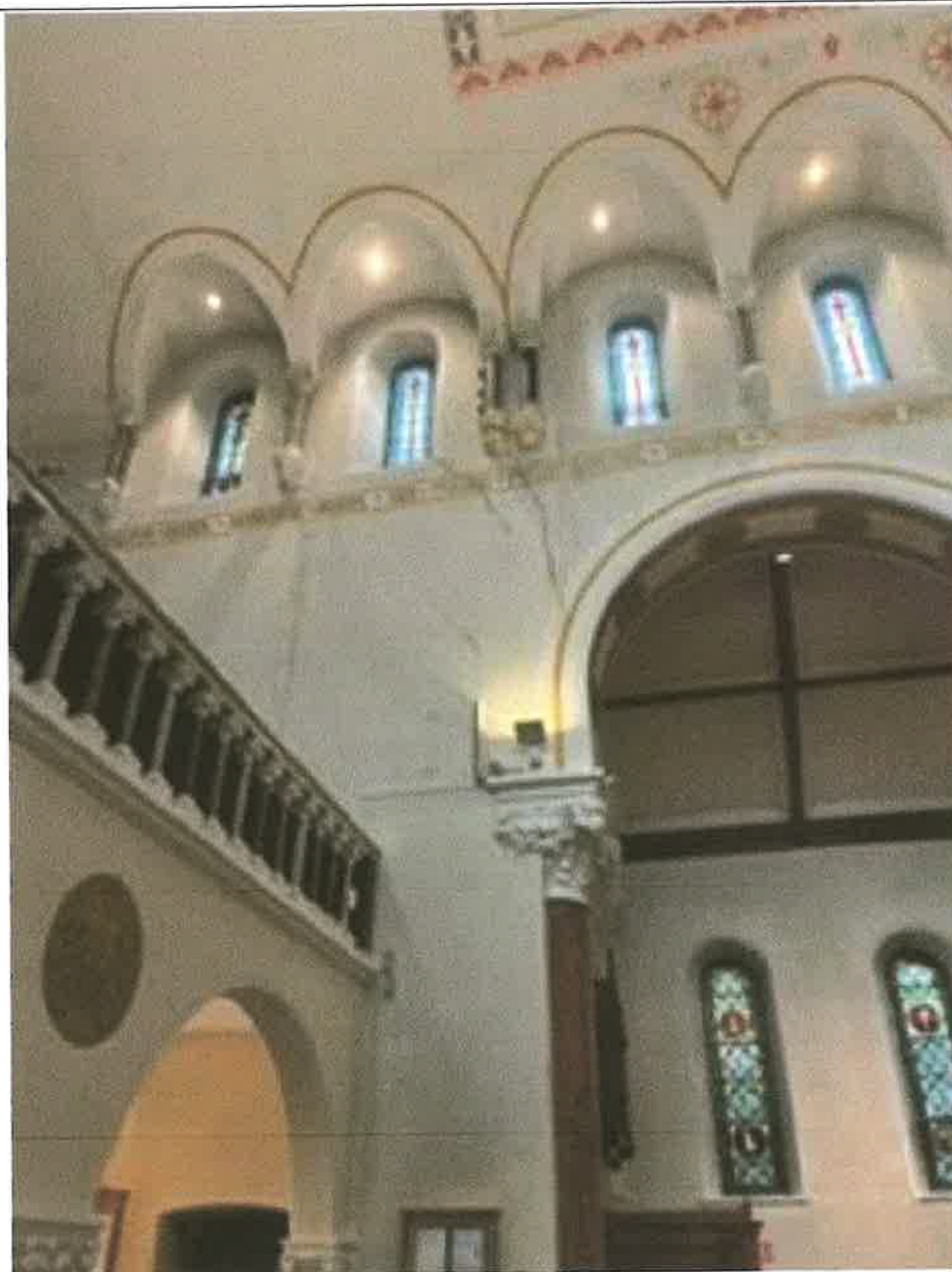
Recent photograph showing deterioration to internal lime plaster at high level on west side of nave (May 2026) This photograph as recorded in the first week of May 2026. The deterioration is linked to saturation of the external masonry at high level, due to the failure of the lightweight copper gutters.
