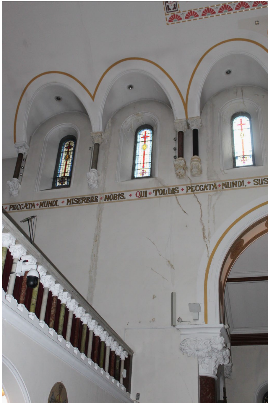
Figure 8: Upper part of south end of interior of east nave wall with significant water ingress damage to plaster wall surfaces and paintwork.
