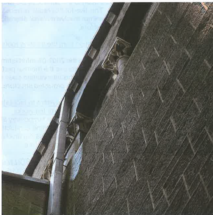
Fig. 7 Existing poor quality pressed copper box-section eaves gutter and square downpipe. Note the modern cement strap pointing on the external façade.
