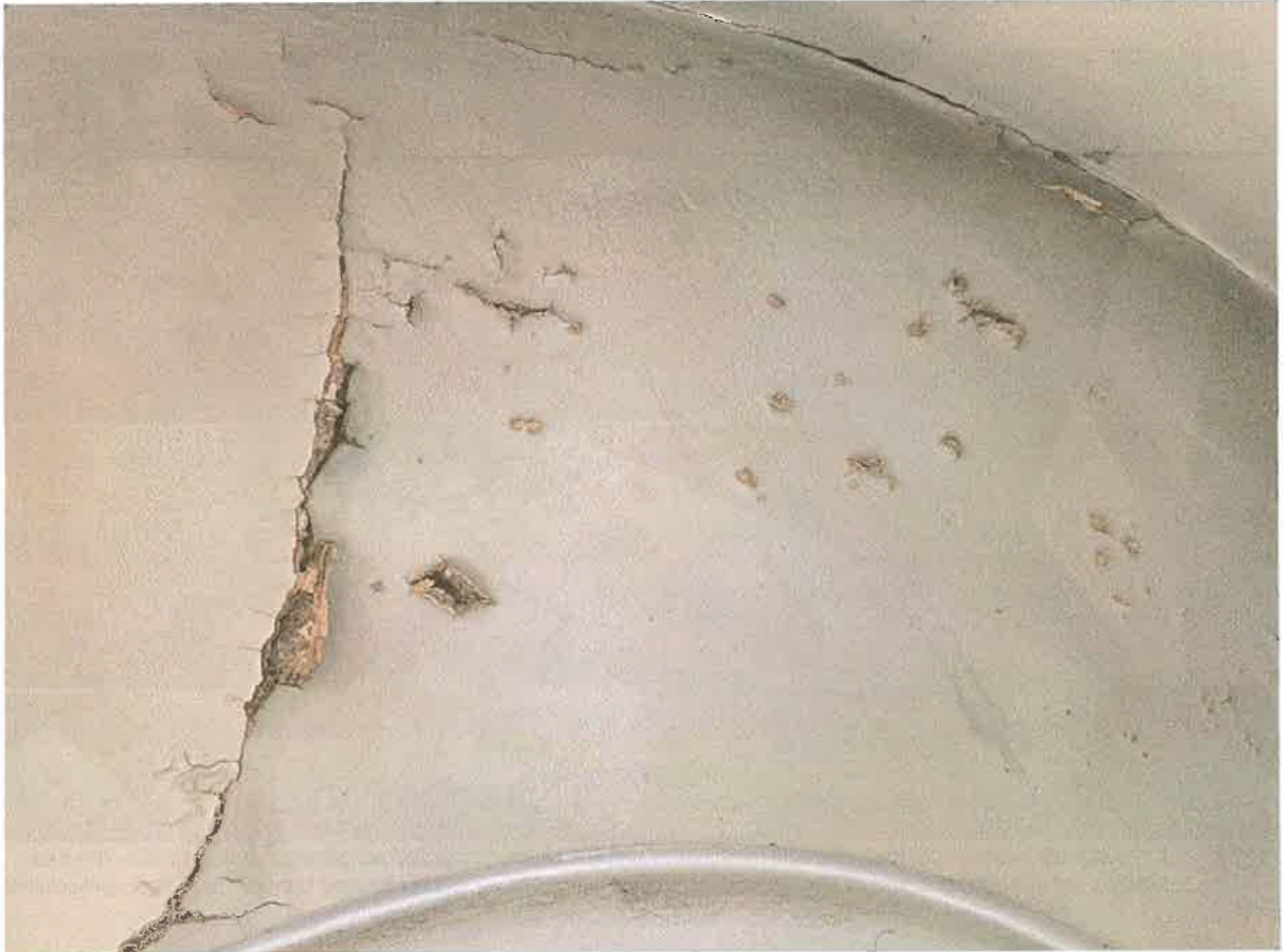
Fig. 8 Damage to internal plasterwork above clerestory window. This damage is due to leaks in the eaves gutter externally, with moisture becoming trapped behind the cement mortar strap pointing.
