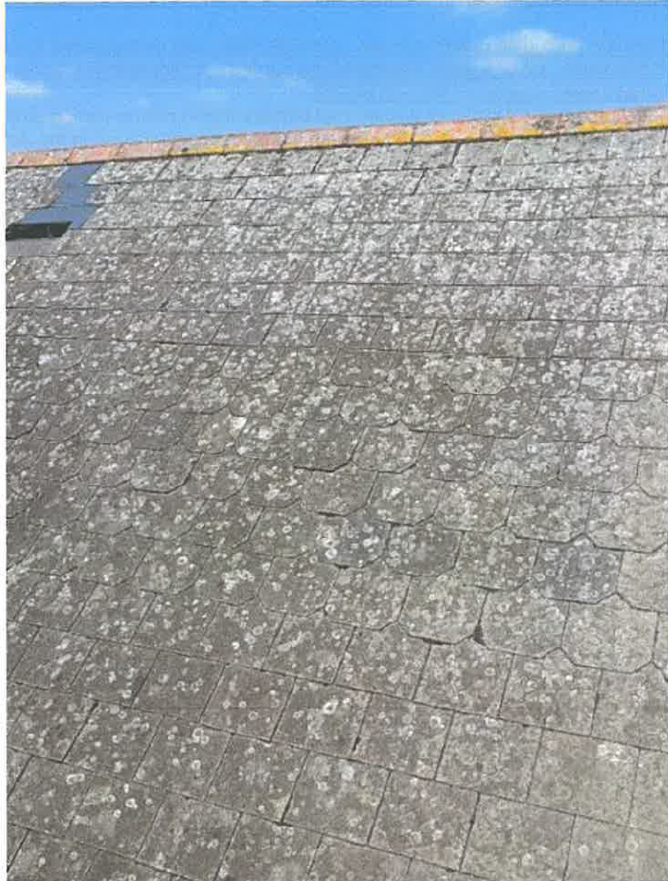
Fig. 5 Detail of west slope of roof showing deterioration in the fibre cement slates
